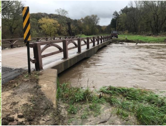
Station Photo down-stream Bridge 8-October 10, 2018 Typical post-storm event with high water and sediment load.
